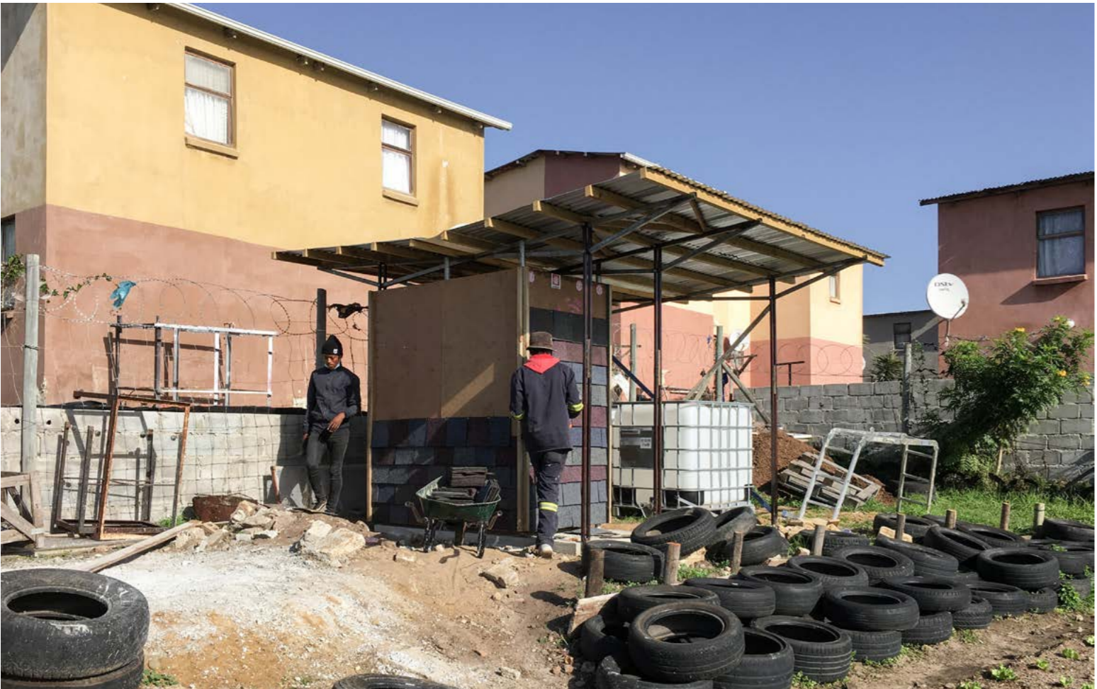
1. 05.20 - Building the roof structure in the workshop © saga 2. 06.20 - Building the roof on site © saga 3. 06.20 - Laying the carpet cladding © saga
